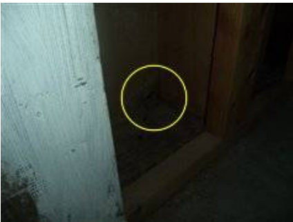
Photo 60-1 Basement bathroom, Behind or inside of wall behind basement kitchen
