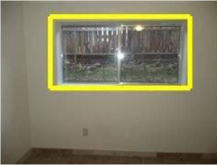
Photo 59-3 Basement, Multiple windows in home
